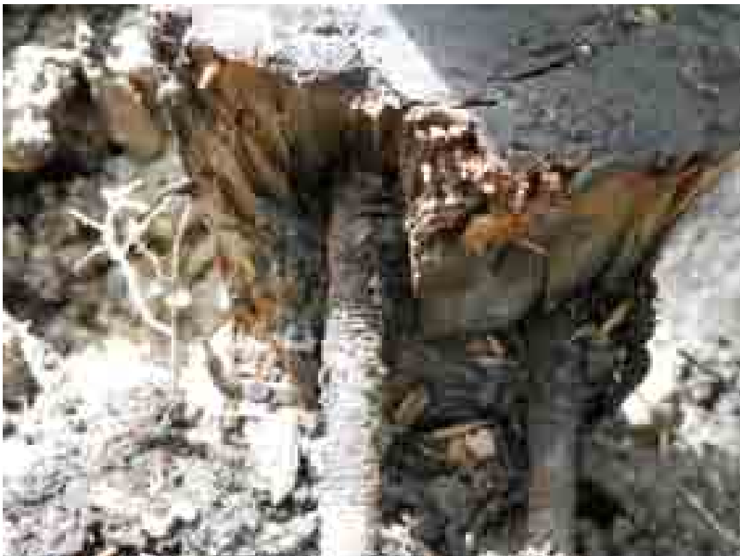
Rotten support block with Coach Bolts
